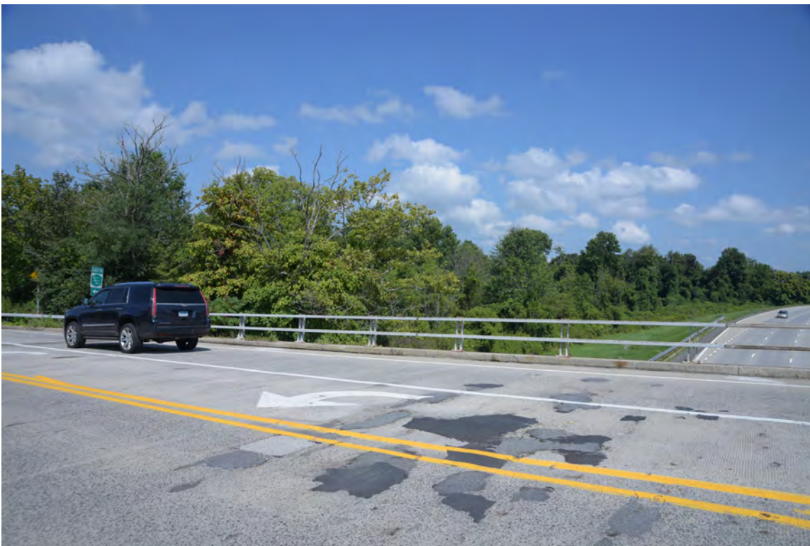
Photo 10 The bridge on Hospital Road passing over Sprain Brook Parkway looking northeast at the Project Site.
